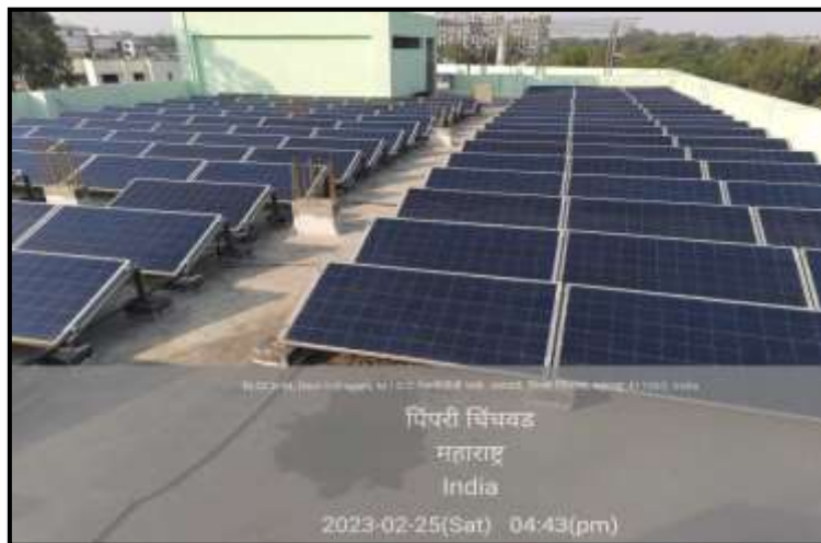
Photograph of Roof Top Solar PV Plant:
