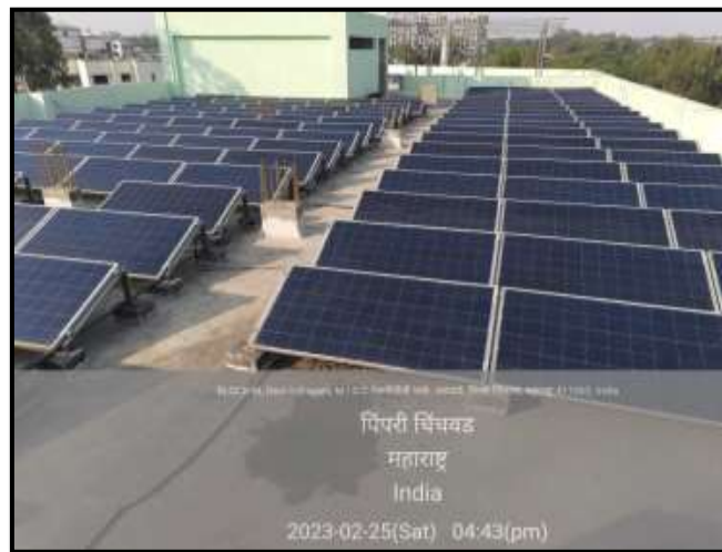
Photograph of Roof Top Solar PV Plant:
